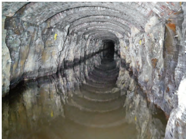
Victorian brick reinforcing arches, added after blasting for the twin-track tunnel damaged the roof. Photo Gerald Tompsett
